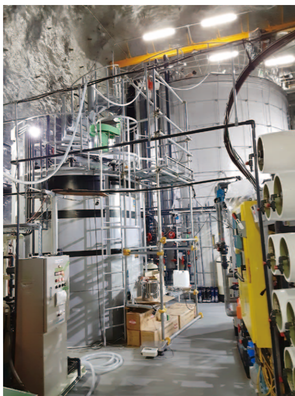
Figure 1: EGADS, the large-scale gadolinium test facility in the Kamioka mine
